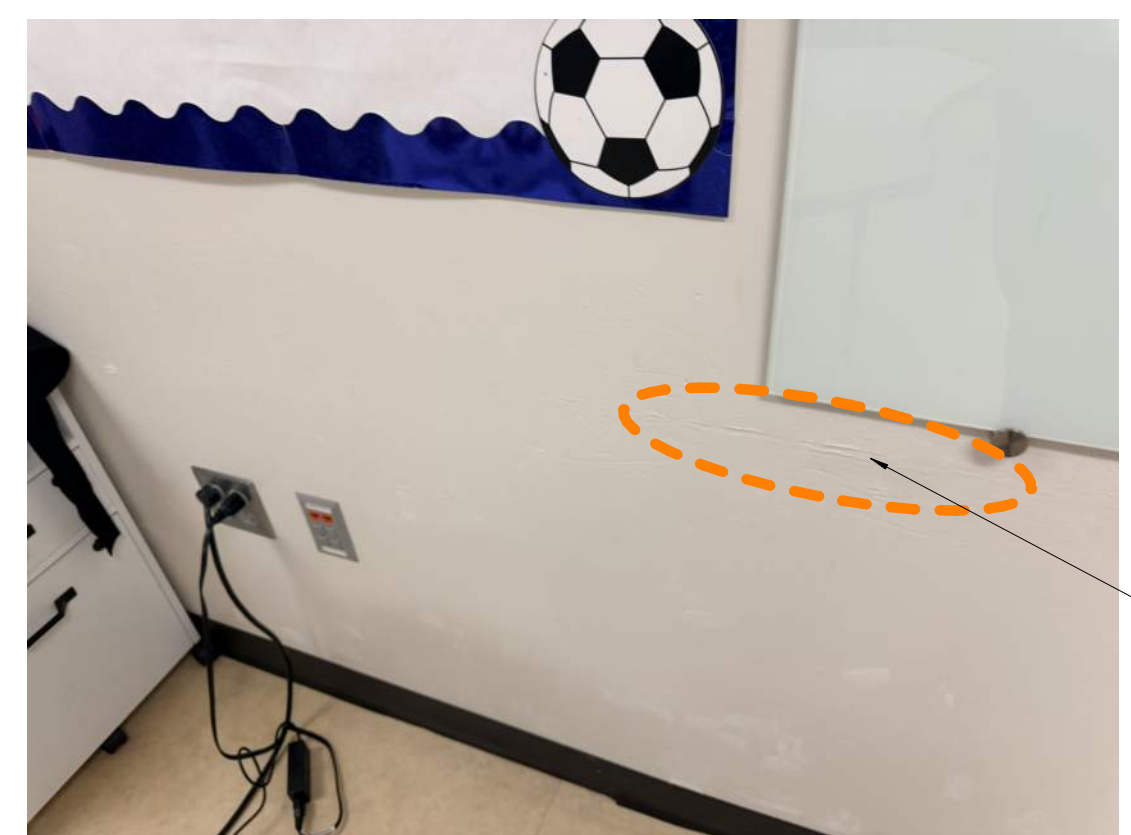
TYPICAL WALL DAMAGE @ CLASSROOM WALLS
